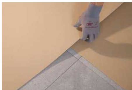
17- Protect the paving against premature loading, other construction work and adverse weather. We recommend covering the paving with sheets or boards to avoid a build-up of dirt and to protect from scratches, abrasion and impact.
